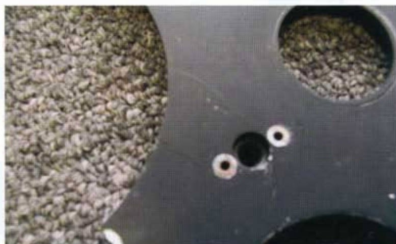
An 8-32 nutplate installed in an oversized hole.
