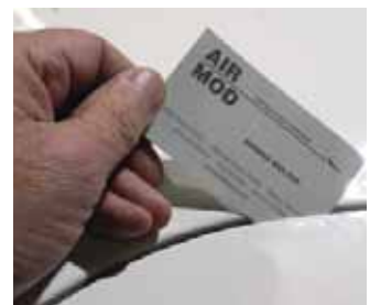
The old business card trick does a pretty good job of finding potential leaks.
